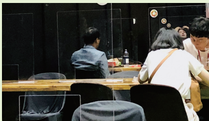
Installation of acrylic shields in a convenience facility of the exhibition hall
